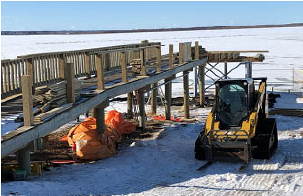
Photo of the platform construction site taken by Miles Constable on March 3 rd
